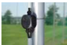
Lighting control of a sports field
